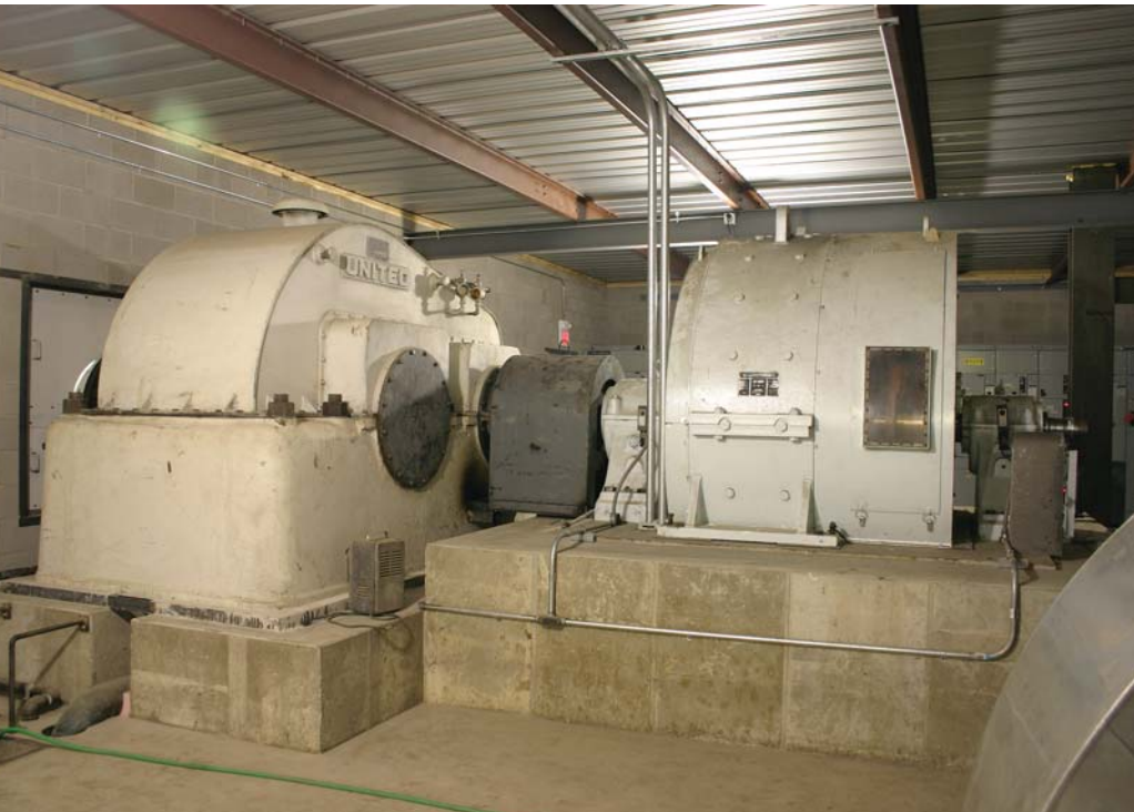
The motor and reduction gear for the 2,000-horsepower mill drive. Each of the two tension reels is turned by a 600-horsepower motor.
