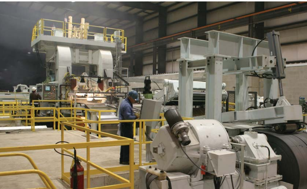
The payoff processor handles coils up to 72,000 pounds and includes a flattener to remove coil set to facilitate strip threading. To be added is a high-pressure washer for hot band that combines a caustic solution with powered brushes.
